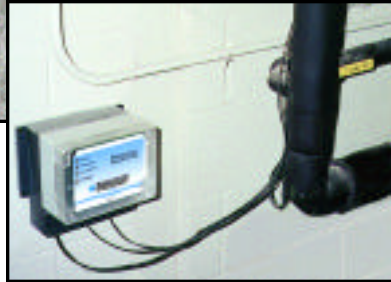
Solenoid wrapped pipe (Coil hidden by insulation) with deposit controller
