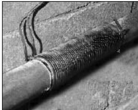
Solenoid Coil wrapped around pipe.
