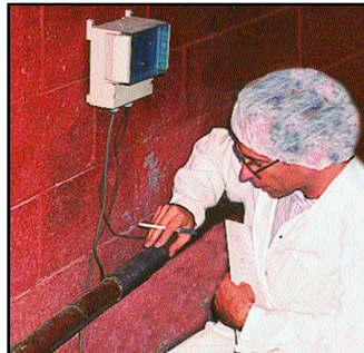
Technician Inspects Triangular Wave Coil and Power Supply
