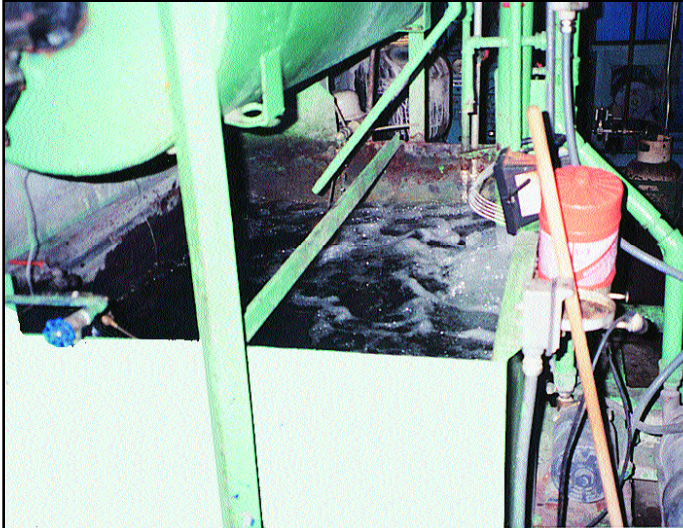
Cooling tower and water holding tank ( shown here ) Old scale detached from the tower
